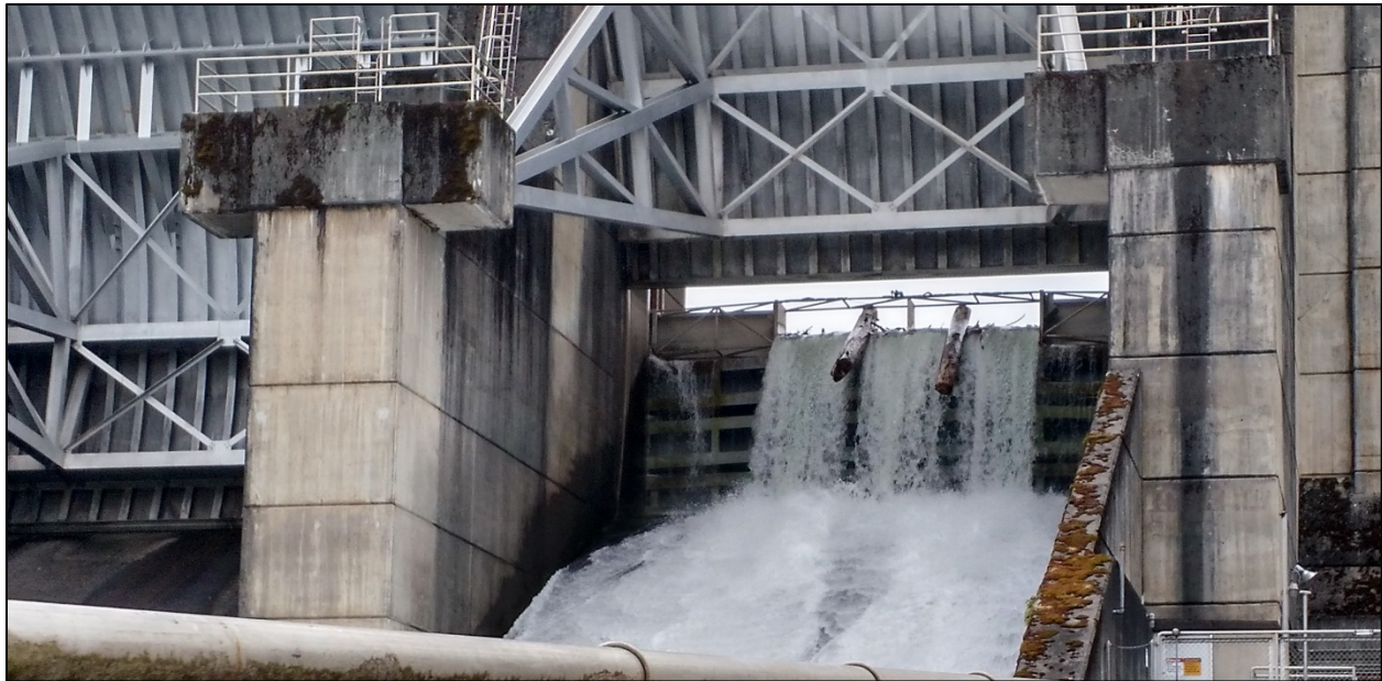
Figure 4-5: Existing weir during operation with logs "see-sawing" through the opening and making contact with top truss.
